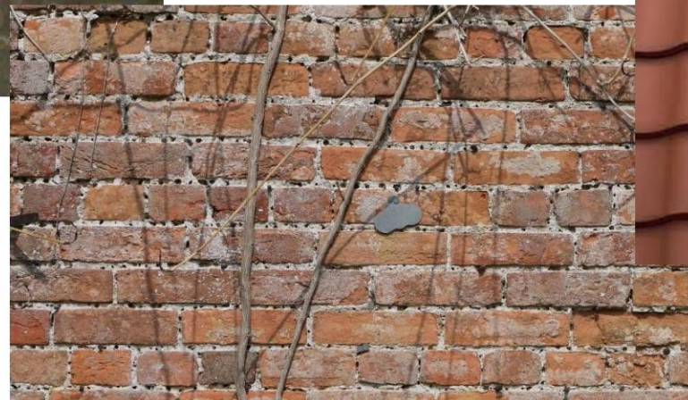
Reclaimed brick to walls of Rebound Room, Central Pool building & below DPC level to plinths of contemporary elements.
